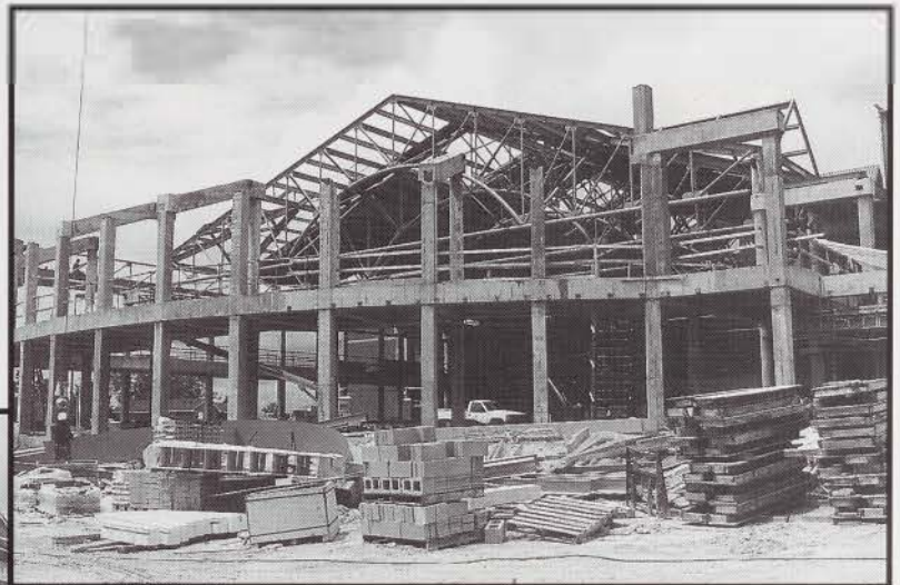
Construction is nearing completion on a new Student Recreation Center, which should be completed in Fall of 1996.
