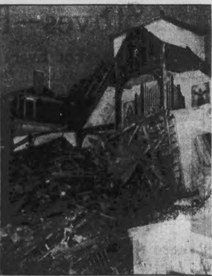
Only a wall supporting the pipe organ remained standing after St. Hedwig's, a Polish church in East Cambridge, Mass., was struck by a hurricane that swept over the New England states. Nearly 500 persons are known to have lost their lives. Damage was estimated in the millions. (Other Storm Pictures on Page 6)
