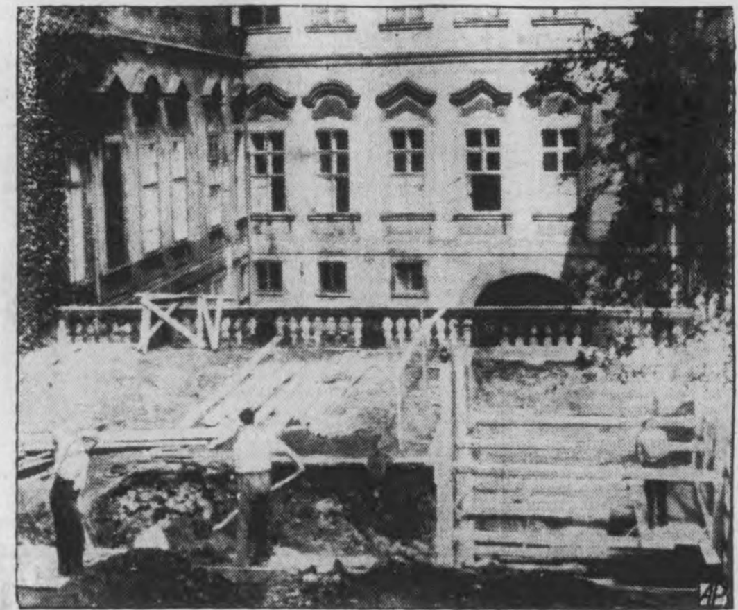
In the garden of the American legation at Prague, Czechoslovakia, is a bomb-proof shelter for use by the staff if war comes. The Czech government approved the precautionary step. Here workmen are shown on the job, with the legation building in the background.
