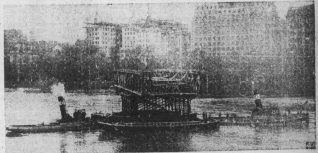
MAN WAITED FOR TIME AND TIDE in setting two 110-ton navigation spans in position near site of the new permanent Waterloo bridge at London. With hawsers steadying them, the spans—one of which is shown resting on barges—sank inch by inch as the tide ebbed until ends of the horizontal girders rested accurately on the greased tops of river piles below.
