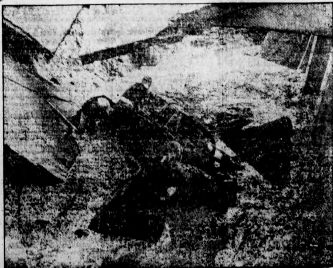
This picture of two smashed ends at the bottom of a wrecked bridge near Del Mar, Calif., graphically illustrates the terrific force with which flood waters of Southern California raged through gulches and lowlands, inundating countless acres, and leaving a death and missing toll of 144 persons. Hapships of concrete, weighing thousands of pounds, can be seen dangerously balanced at the top of the bridge.
