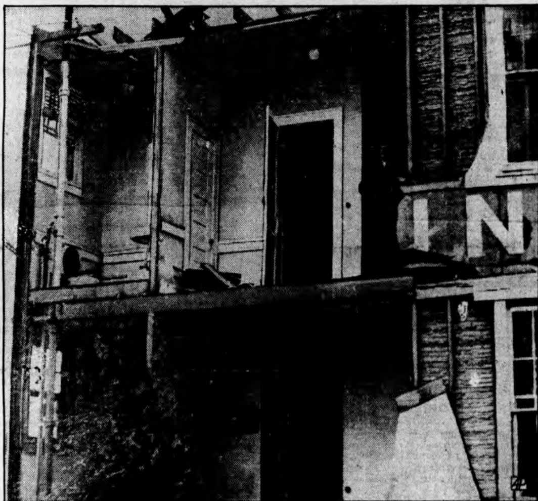
HOLDING OPEN HOUSE IN MOBILE was unintentional but forceful when a twisting wind storm struck that Alabama city's waterfront, leaving several persons injured and heavy property damage in its wake. Here's one of the homes in the path of the storm, its rooms left exposed when walls were blown away. The gentleman gazing from the second floor seems unperturbed by the open-air vista spreading before him.
