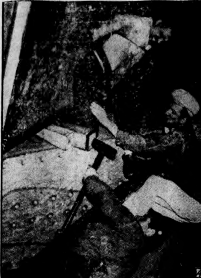
His leg crushed under a two-ton pier door which fell and trapped him on a construction job in Boston. Frank J. Downes, army base electrician, directed his own rescue while fellow workers tried desperately to lift the door. Note the look of agony on his face and the wedges driven under the door in efforts to lift it.
