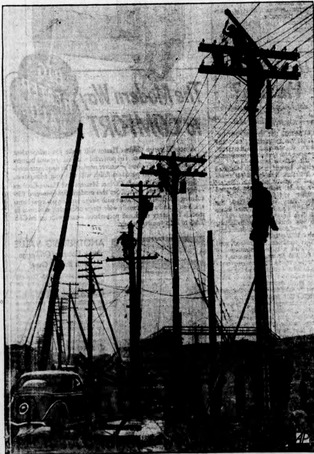
A TOOTHACHE THAT HALTED INDUSTRY was reported by Buffalo's Police Lieutenant William Marnon. As Halbert I. DeFreest drove home after having his teeth extracted, he felt faint, pulled his car to the curb, hit a power pole. Eleven other poles were pulled down, street and house lights went out, a standard exploded, 4,000 men in eight factories were made idle and 200 line-men worked 12 hours to straighten things out.
