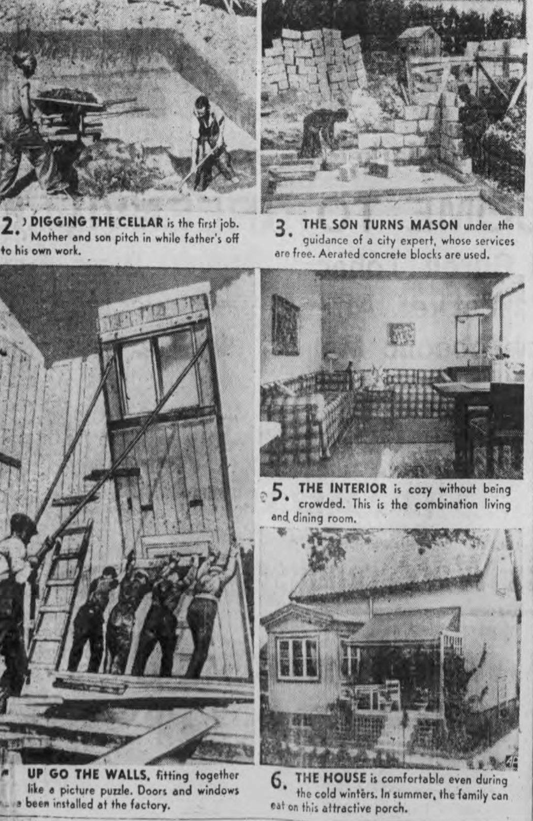
1. THE SITE was selected in this attractive Magic House colony. Note the attention paid to roads, and the fair-sized plot allotted each family. 2. DIGGING THE CELLAR is the first job. Mother and son pitch in while father's off to his own work. 3. THE SON TURNS MASON under the guidance of a city expert, whose services are free. Aerated concrete blocks are used. 4. UP GO THE WALLS, fitting together like a picture puzzle. Doors and windows have been installed at the factory. 5. THE INTERIOR is cozy without being crowded. This is the combination living and dining room. 6. THE HOUSE is comfortable even during the cold winters. In summer, the family can eat on this attractive porch.
