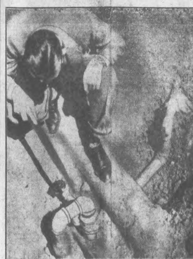
This exclusive picture shows where New London, Tex., school officials made an unauthorized plug-in on an oil company's waste gas line for free fuel which some believe caused the explosion that killed 453. The man is pointing to the small pipe tapping the main line. An explosions expert said the blast was caused by gas accumulated under the school basement floor. (Associated Press Photo)
