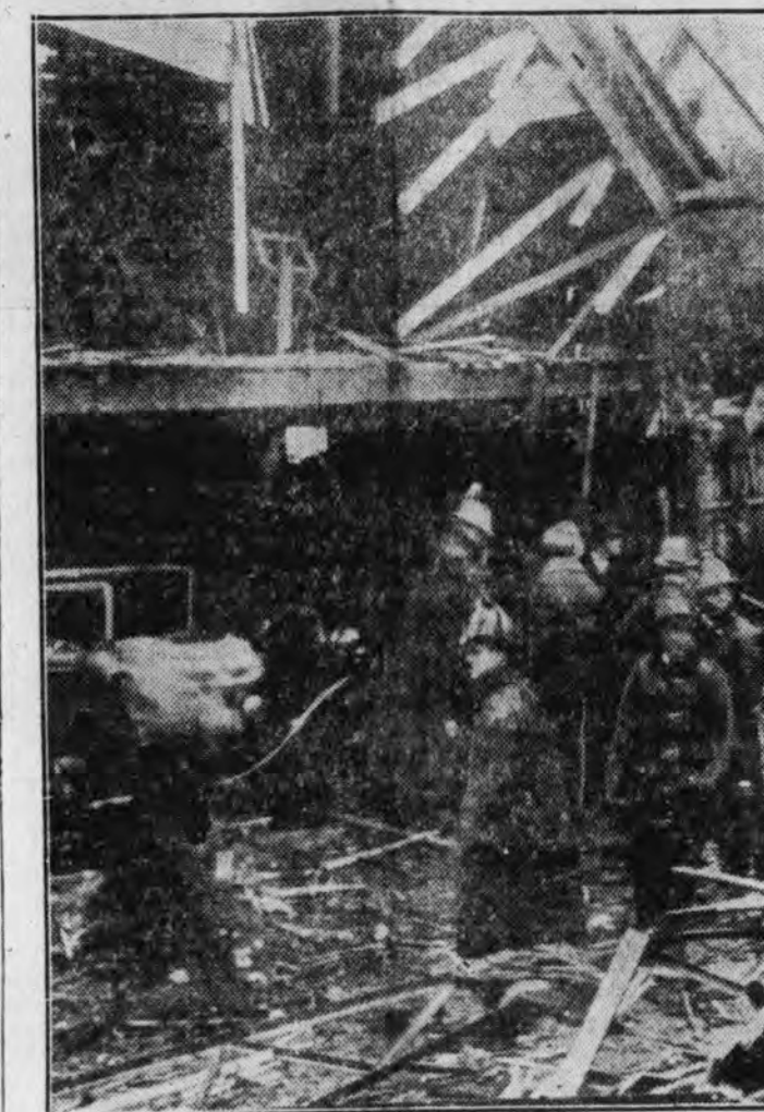
A mysterious series of bombings that spread terror in Milwaukee finally came to a climax with a terrific explosion in a garage that killed three persons and injured eleven. This picture shows the wrecked building which police believe was used by the bombers as a storage room for their dynamite. (Associated Press Photo)
