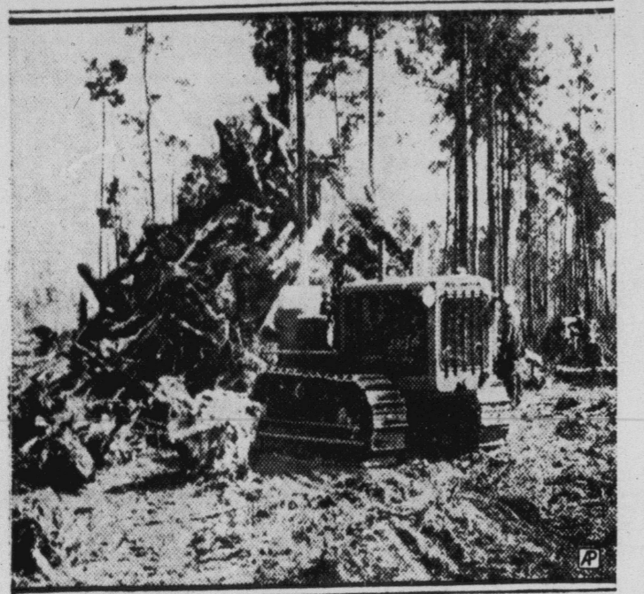
This is a scene at "Penderlea" Pender County, N. C., where 4,500 acres have been set aside for a subsistence homestead project. Giant tractors were used to clear the land of tree stumps. It is planned to settle some 400 families there.
