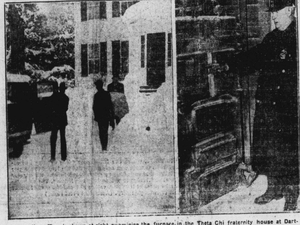
A police officer is shown at right examining the furnace in the Theta Chi fraternity house at Dartmouth where nine students died of carbon monoxide poisoning while they slept. Investigation revealed that a slight explosion had broken the flue pipe and allowed the gas fumes to penetrate the upper floors of the house. Picture at left shows authorities removing the body of one of the victims. (Associated Press Photos)
