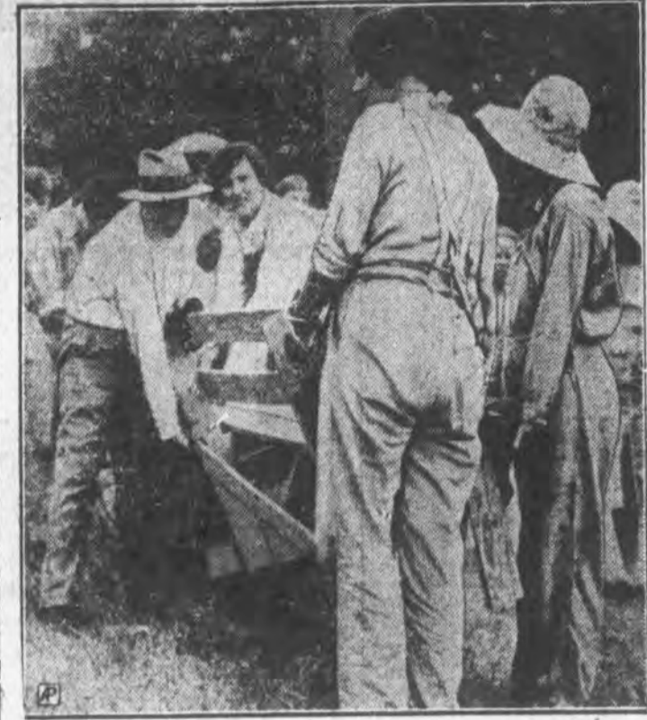
Women took over the construction of a fundamentalist Baptist tabernacle in Dallas, Texas, after the court issued an injunction halting "men" from working on the building at the request of adjacent property owners. The women worked night and day shifts on the building.
