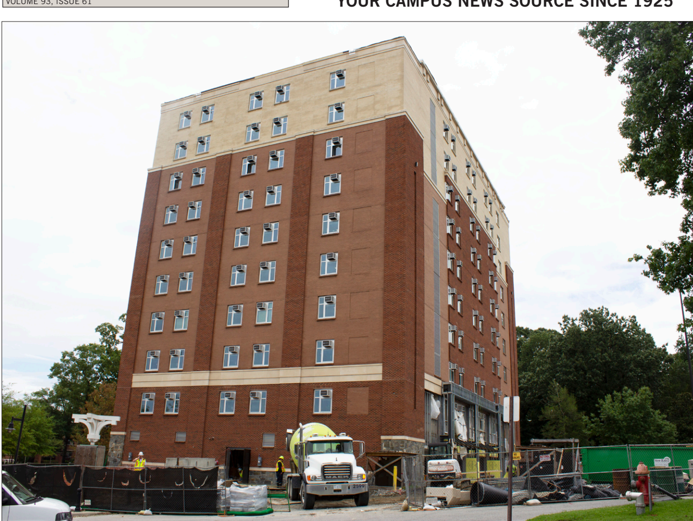
West End's Greene Residence Hall renovations began in May 2018 and are scheduled to be completed on time, as planned for fall 2019.
