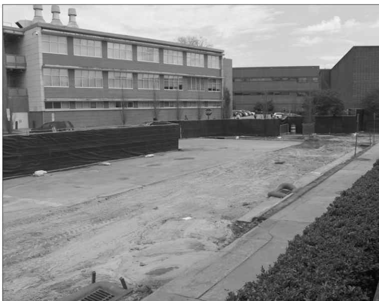
Construction in front of the Slay due to the issues with the steam system.
