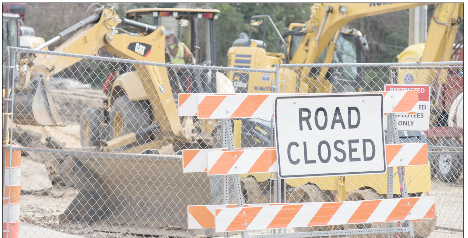
Construction continues on the Town Creek Culvert that will assist with storm water draining in the Uptown area. Construction began last spring.
