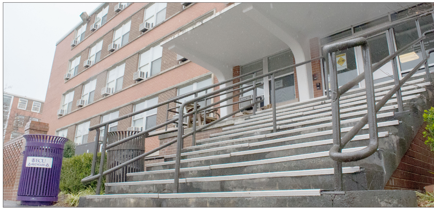
The stairs of Legacy Residence Hall where students living in the building have reported both mice and mold, creating tenuous living conditions.
