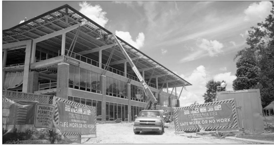
Construction continues on East Carolina University's new student center, which will open Jan. 7.
