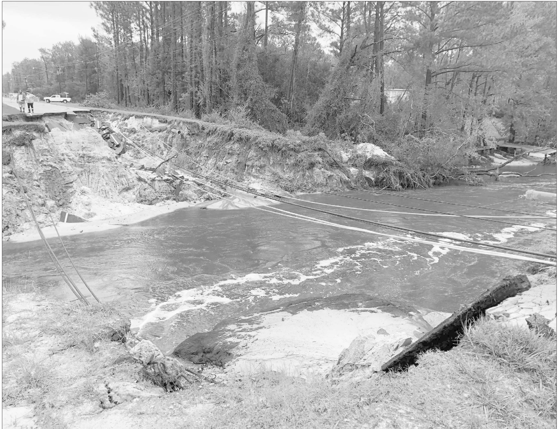
A roadway was washed away by Hurricane Florence in the Boiling Springs Lake, North Carolina area. Hurricane Florence brought record amounts of rain to parts of the state already soaked.
