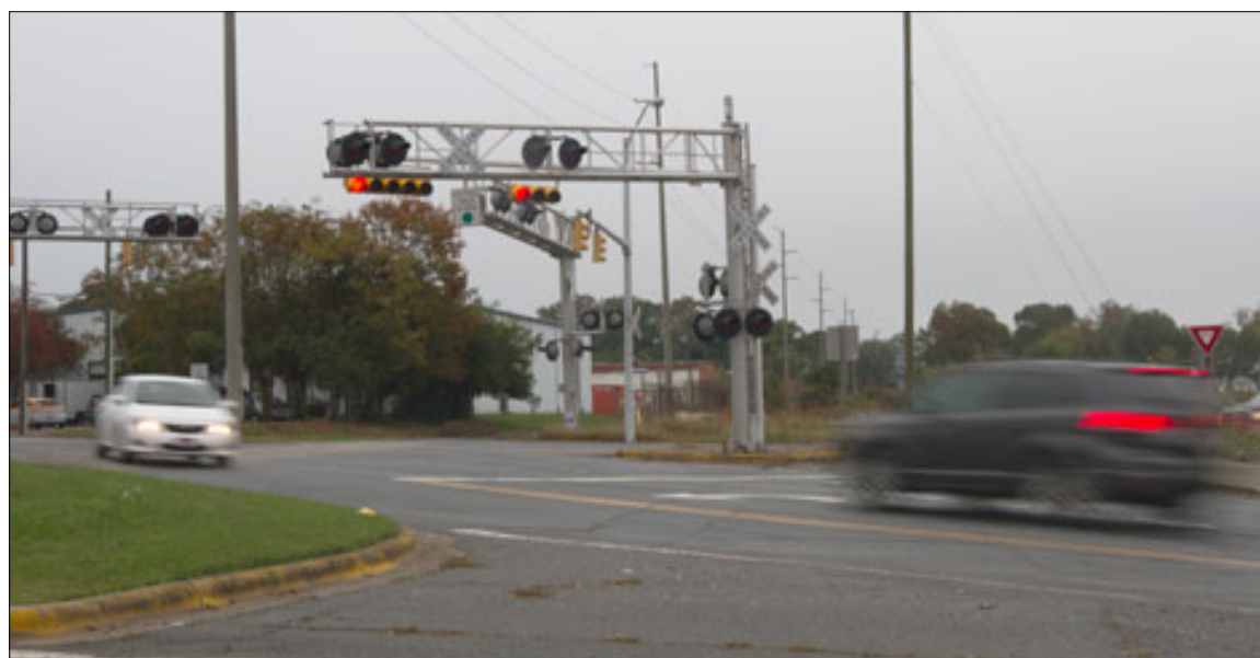
At 10th Street and Dickinson Avenue, the new road will elevate over the railroad tracks. Construction will begin in March.
