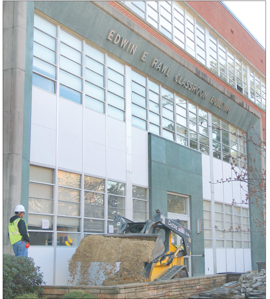
Construction workers outside Rawl building work to improve the building for the disabled.
