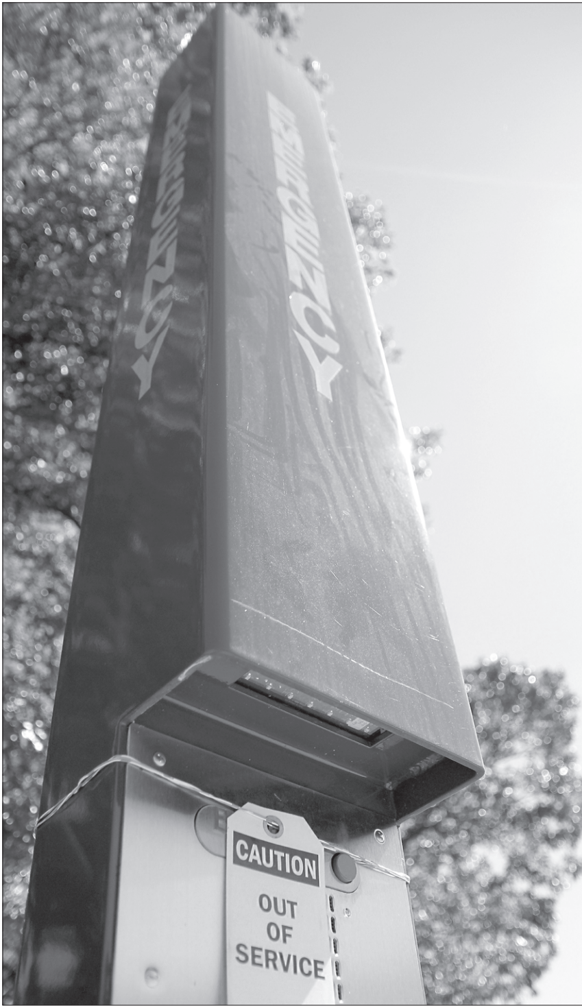
One of the blue light emergency phones at Minges Coliseum is currently out of service. MICHAEL SEEGARS | THE EAST CAROLINIAN
