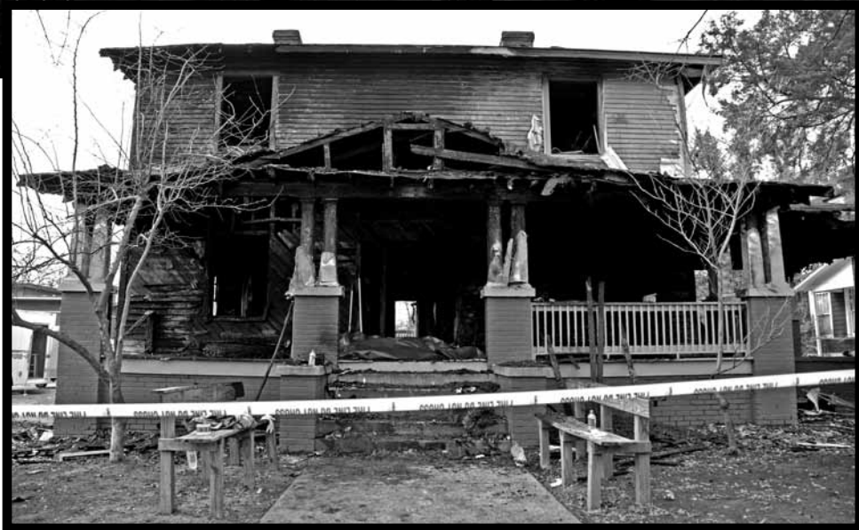
The Sig Ep backhouse reopens Friday August 21 after being completely rebuilt following a fire that destroyed the house in January.
