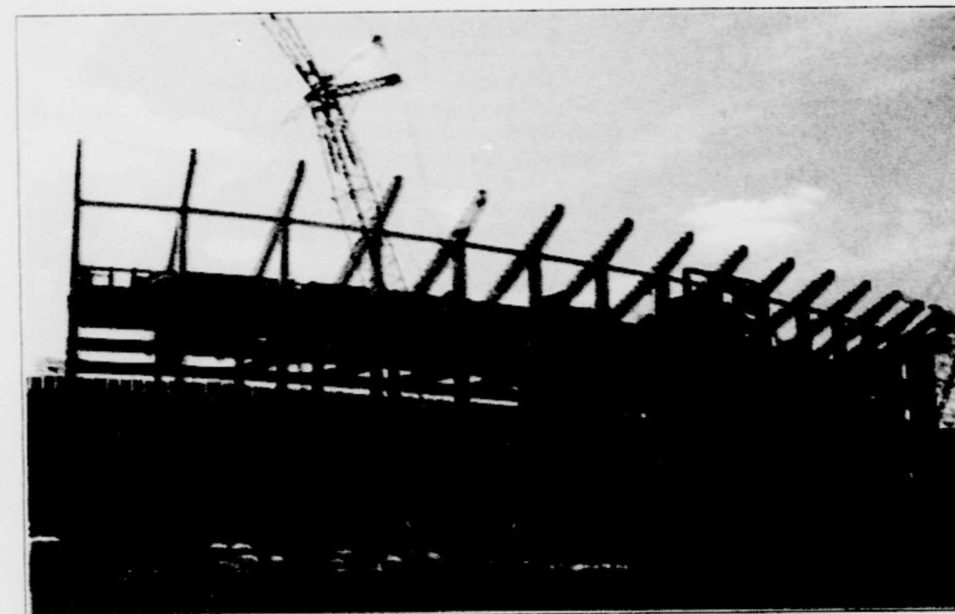
The upper deck expansion, which was supposed to be finished in time for the first home game, is still in progress.
