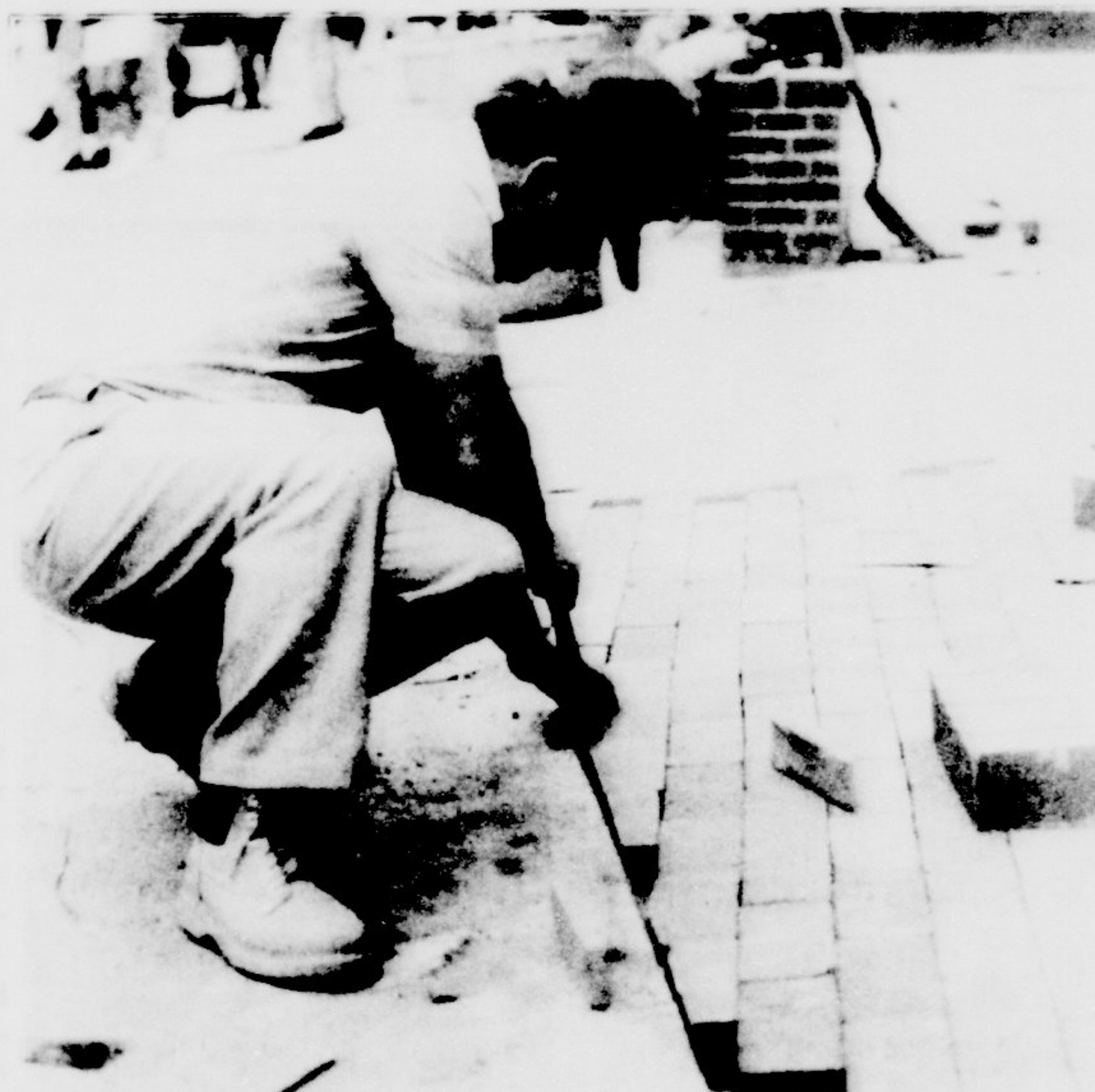
Renovations at the Wright Soda Shop began last week as workers laid bricks for an outdoor eating area
