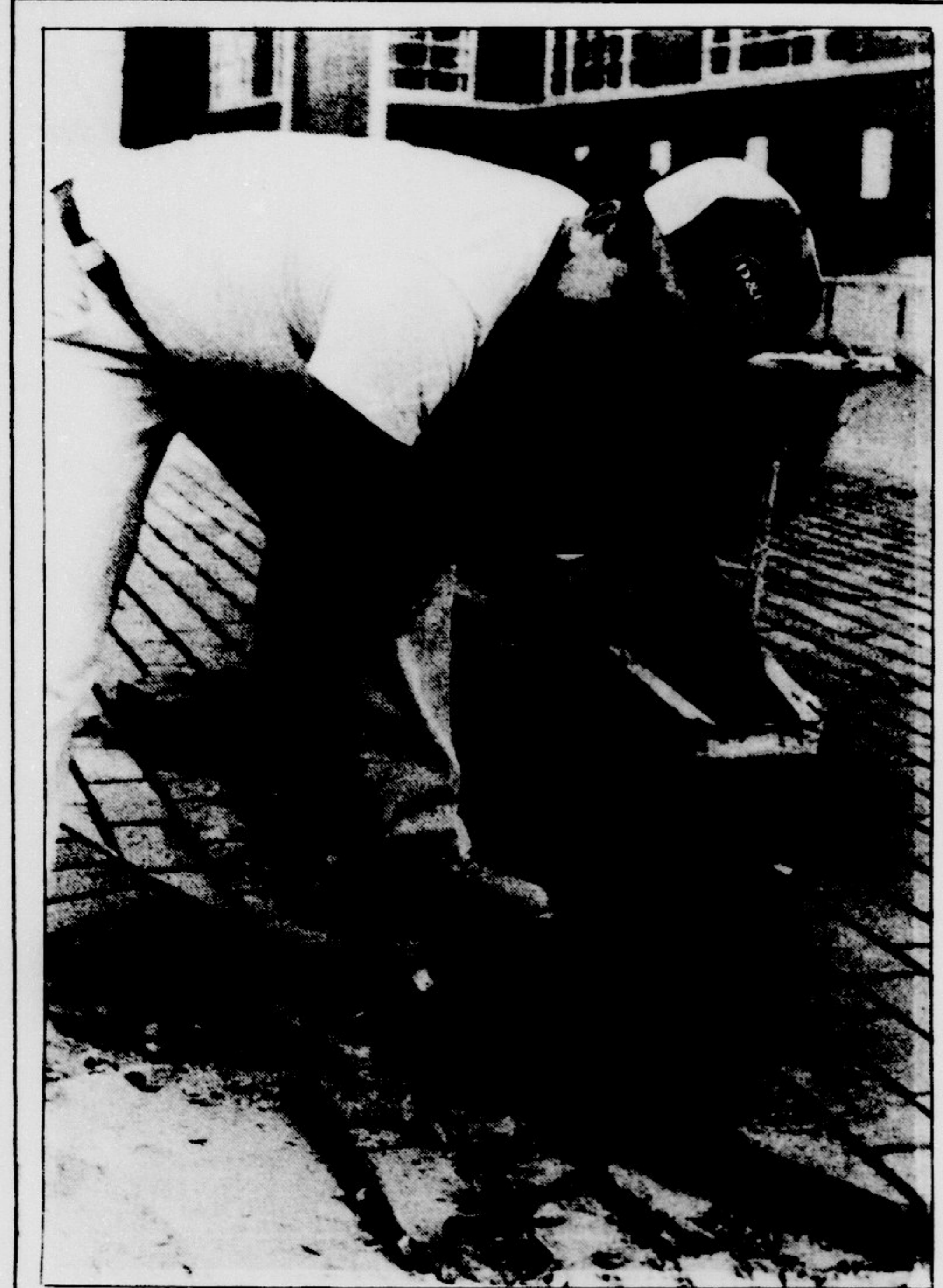
Worker takes a break from sidewalk-building to smile for the camera. (Photo by Matthew Bulley — ECU Photo Lab).
