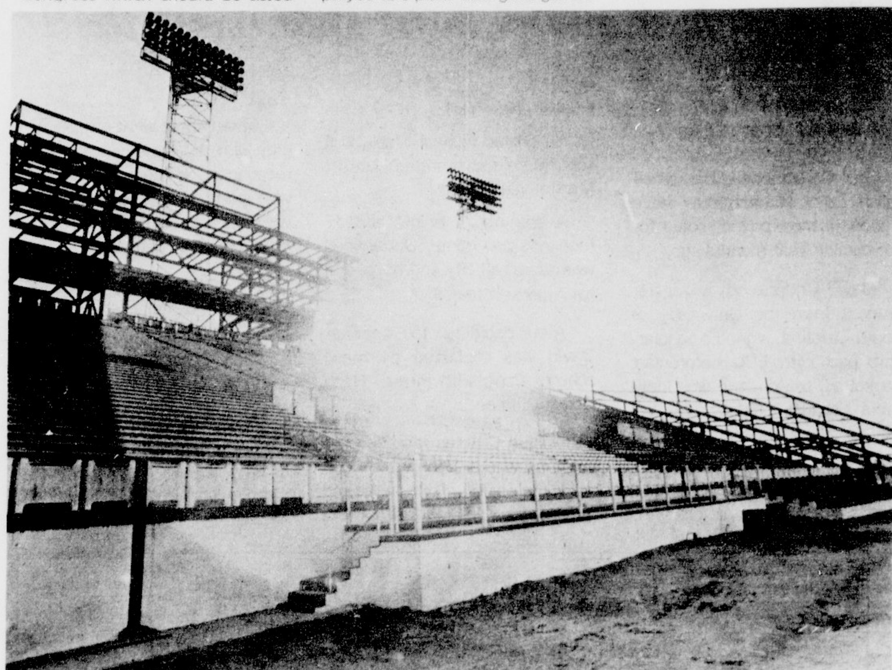
THE SUN SHINES through new steel superstructure of Ficklen Stadium. The expansion is well underway and work should be completed by the fall. Ficklen will hold 35,000 and be North Carolina's fourth largest stadium. [Photo by Brain Stotter]
