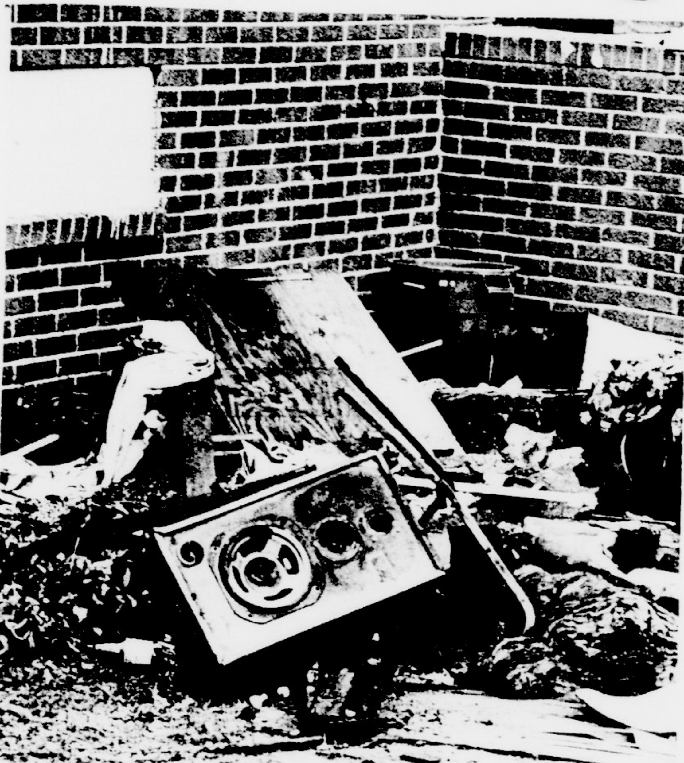
Fire caused major damage at the Tau Kappa Epsilon fraternity house Saturday morning, leaving little more than burnt rubble in many areas of the house. The structure had to be condemned because of the damage.
