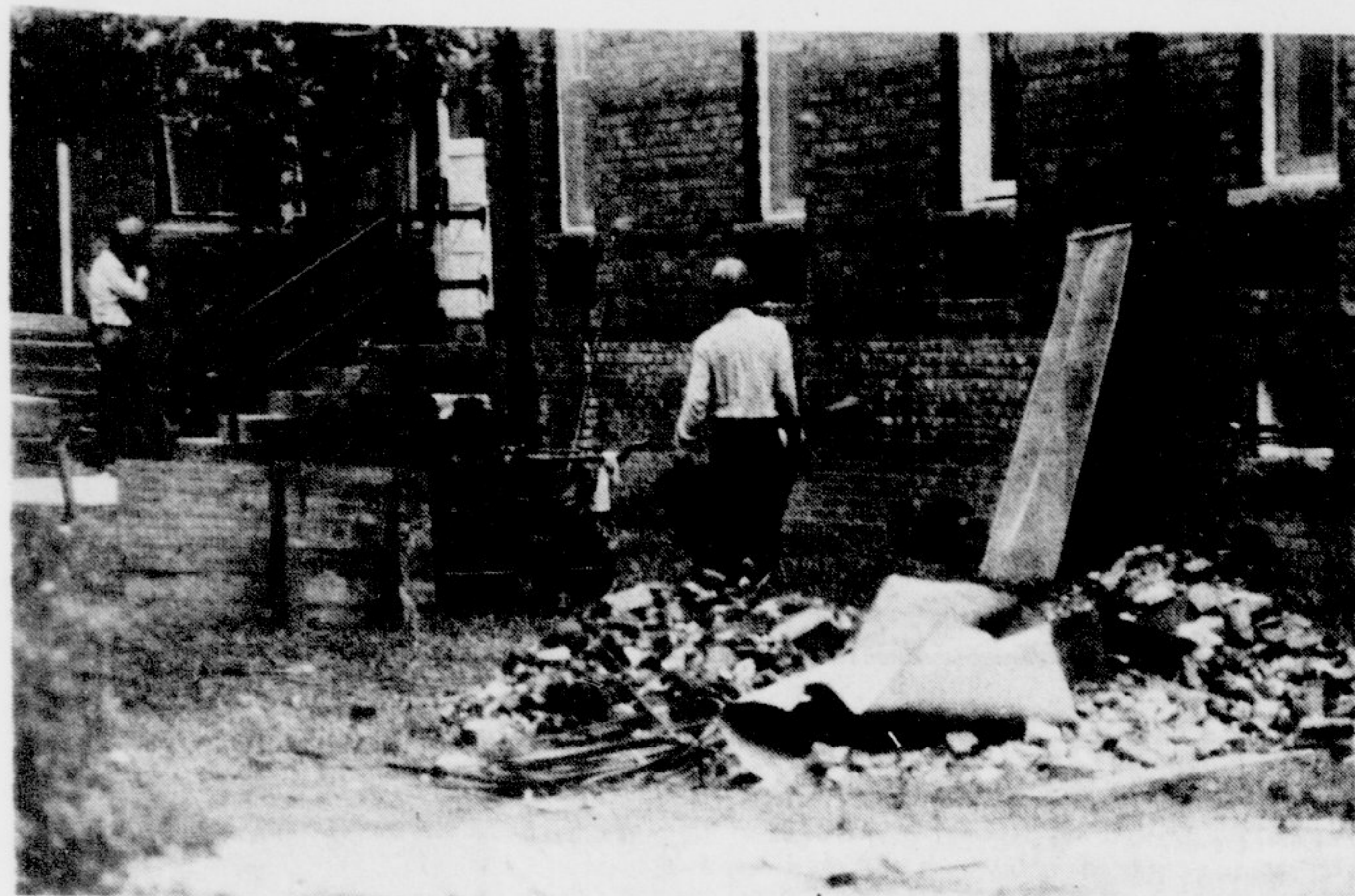
Construction workers labored throughout new look, and residents there are the summer to give Jarvis dormitory a generally pleased with the result. (Photo by John H. Grogan)
