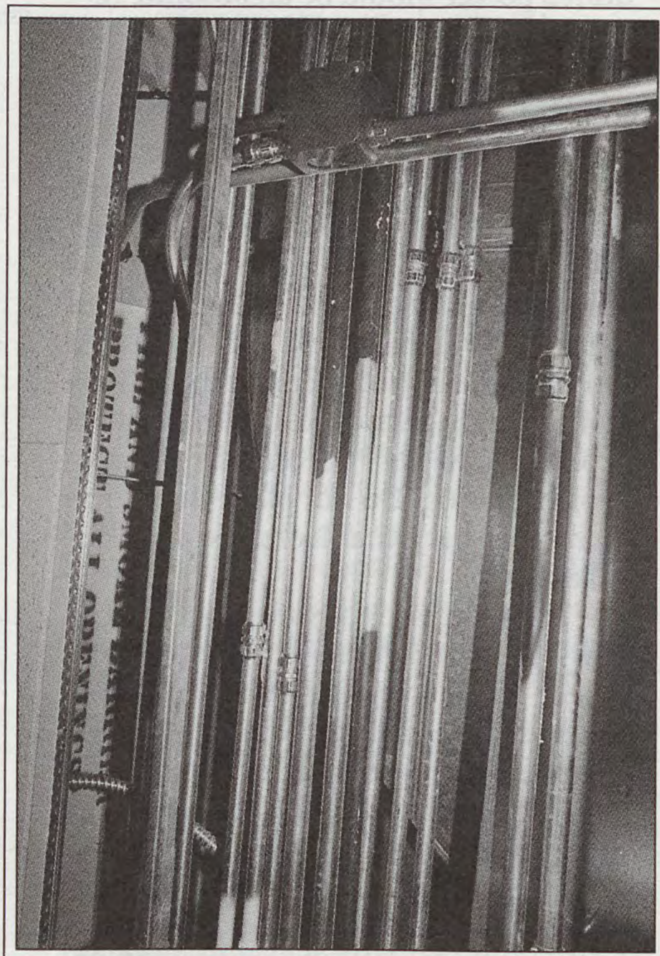
The amount and size of conduit should not be underestimated. (Photo: Joyner Library, East Carolina University.)
