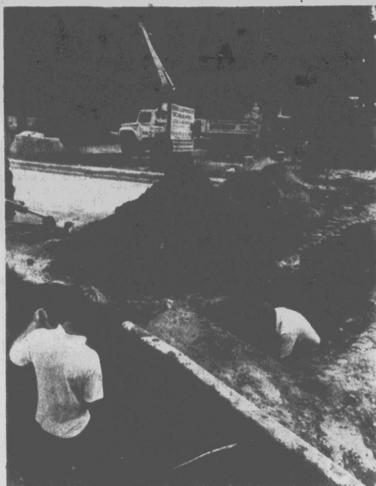
POWER FOR BUILDING — Jeff Gay, left, and Ronnie Whitley complete work on a trench leading to the new general classroom building being constructed on the East Carolina University campus. The trench will carry the primary electrical lines to the building. (ECU News Bureau Photo By Tony Ruple)
