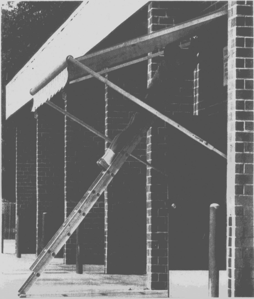
At AN ANGLE — Glenn Swanson holds on with a confidence that others might say had a shaky foundation. He was on the sharply angled ladder at the car wash at the corner of Evans and 10th streets while replacing conduit tubing. (Reflector Photo by Cliff Hollis)
