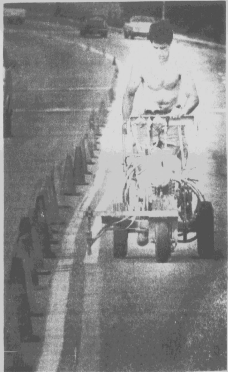
UPHILL ALL THE WAY — Bob Blick walks up College Hill Drive while repainting the center line. Blick was with a crew that painted new lines in the parking lots and streets around East Carolina University dorms Monday afternoon. The painting is done every summer after the spring semester ends. (Reflector Photo by Cliff Hollis)
