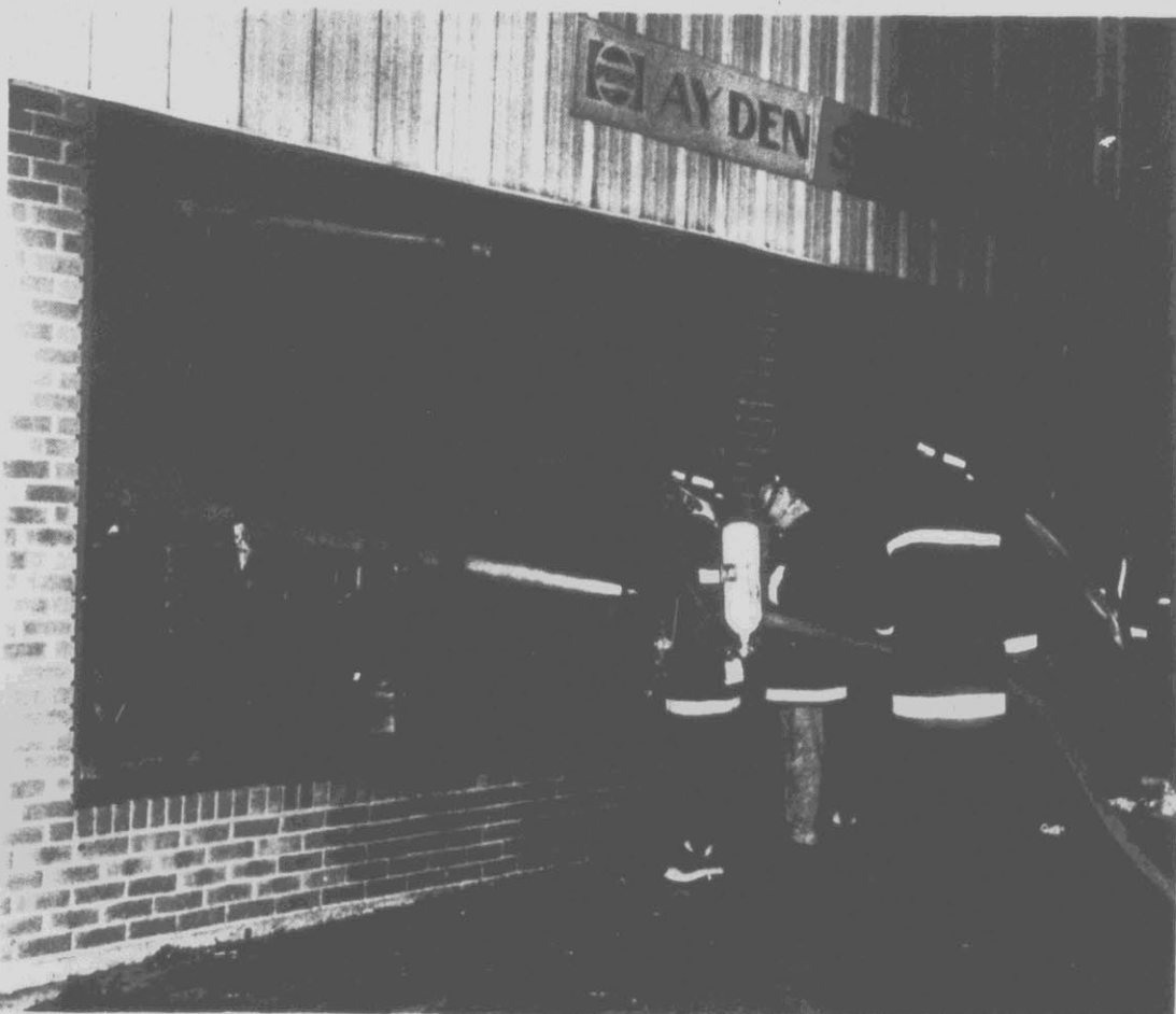
BUSINESS DAMAGED — The Ayden Sport Shop on 312 East Ave. in Ayden was heavily damaged by fire Monday. Ayden Police Chief Tommy Burney said the fire was discovered by a police officer about 9:45 p.m. When firemen arrived the front of the building in the showroom area was engulfed in flames. Firemen from Ayden and Winterville brought the blaze under control in minutes, but the building sustained heavy fire, smoke and water damage. Burney said the building, which was owned by Poe and Bill Worthington, was valued at about $100,000. The cause of the fire is under investigation by Ayden police. (Reflector Photo by Tommy Forrest)
