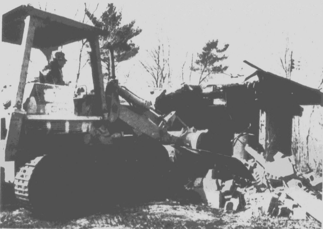
WELL CLOSED — A bulldozer crumbles a building housing one of the contaminated drinking water wells in Woburn, Mass., on Wednesday. The wells have been closed since 1979 due to chemical contamination. Woburn
