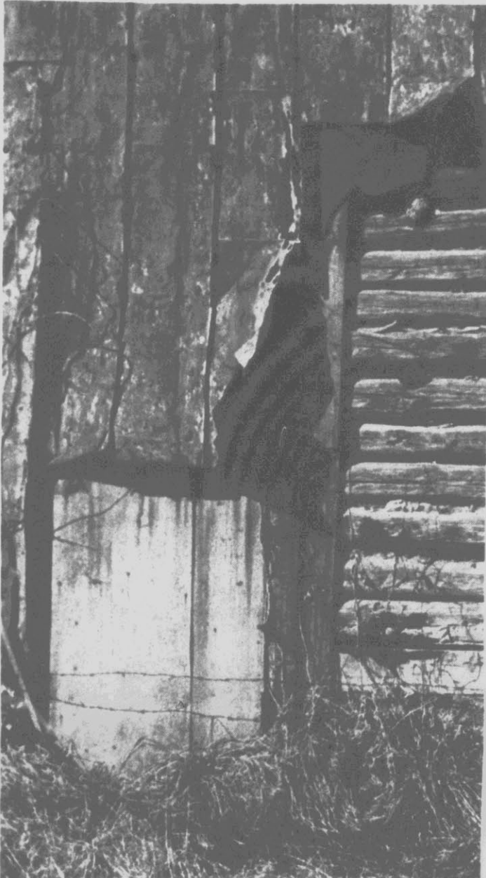
HISTORY REVEALED — The past history of outer coverings of this Pitt County barn northeast of Farmville is told graphically in the barn's corner. The original jointed log construction was first covered with green tar paper and later with tin. Other than this corner, the rest of the barn remains tin-covered. (Reflector Photo by Jerry Raynor)
