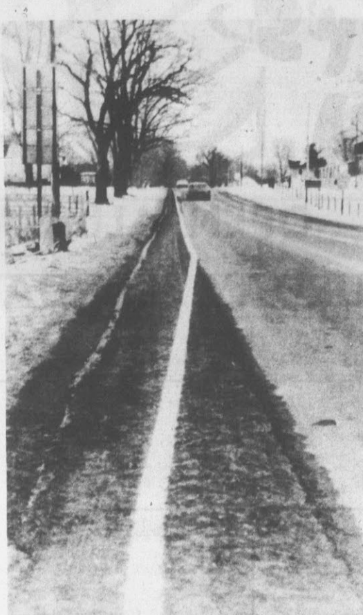
OR-F-COURSE LINE — A white line intended to mark the highway's boundary strays off the pavement of a Crawford County roadway near Meadville, Pa., after a Pennsylvania Dept. of Transportation line-painting crew laid the line on dirt and snow covered shoulder Dec. 6. Several miles of white line missed the pavement, and ended in dismissal of two of the line-painting crew, and reprimands for their superiors this week. (AP Wirephoto)
