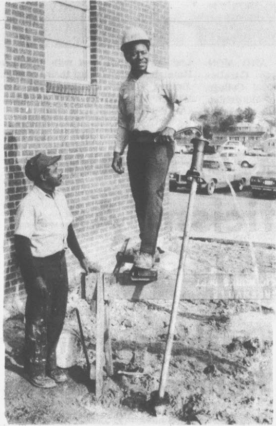
AN UNLIKELY PLACE... for a hand pump, it would seem, is the 200 block of East Third Street, but Greenville Public Works employee Frank Jones spent much of Friday afternoon welding its handle. He said there was an underground water tank that had to be emptied and removed before the sidewalk could be laid. His co-worker Braxie Cox (left) assisted. (Reflector Photo by Carol Tyler)
