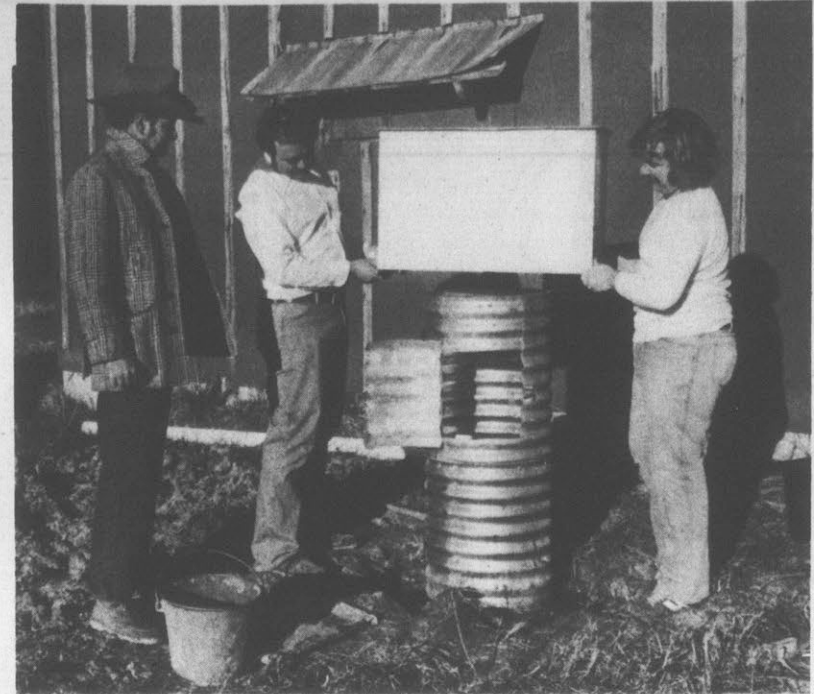
INSTALL OBSERVATION WELL — James Galloway, left watches Gene Baker, center, and Joe Riggsbee, right, hydrologic technicians, install
