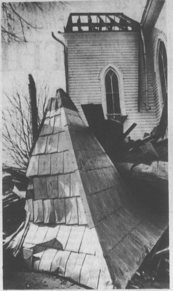
LAST DAYS FOR OLD CHURCH . . . The 153 year old Friedberg Moravian Church here is being torn down to make way for a more modern, larger building. Some parts of the old structure will be salvaged for the new church. (AP Wirephoto)
