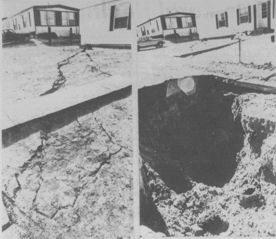
GOING, GOING — Cracks in the dusty front yard of a mobile home in Rock Springs, Wyo., at left, can lead to holes so deep that underground pipes are un-
