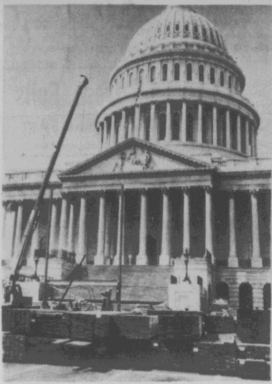
GEARING UP — Workmen start construction of the presidential inaugural stand on the Capitol grounds yesterday. Even though the inauguration isn't until January 20, work is already underway. (AP Wirephoto)
