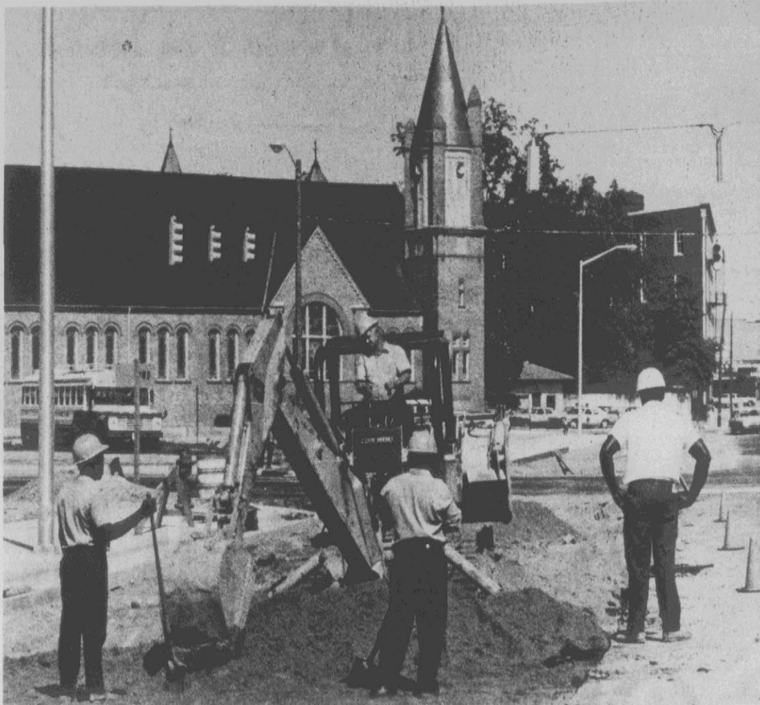
EVERY WORKER HERE IS WORKING TO WIDEN, REPAIR, REPAVED AND IN GENERAL IMPROVED, MOTORISTS ARE CONSTANTLY FACED WITH A CHANGING SERIES OF TEMPORARY OBSTACLE COURSES. RECENTLY, DICKINSON AVENUE HAS BECOME THE MOST AC-
