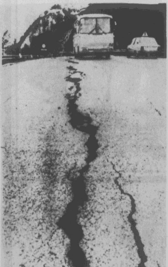
QUAKE-CRACKED ROAD — A crack, several inches wide, and others are clearly visible on the asphalt of a highway at Venzone, in Italy, after new strong tremors hit northern Italy last week. (AP Wirephoto)
