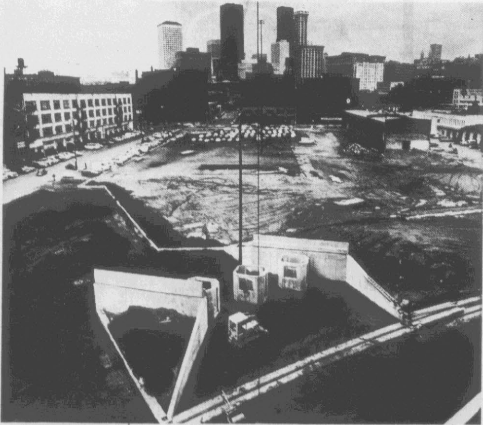
Kingdome's ticket booths take shape, with skyline of downtown Seattle in the background.
