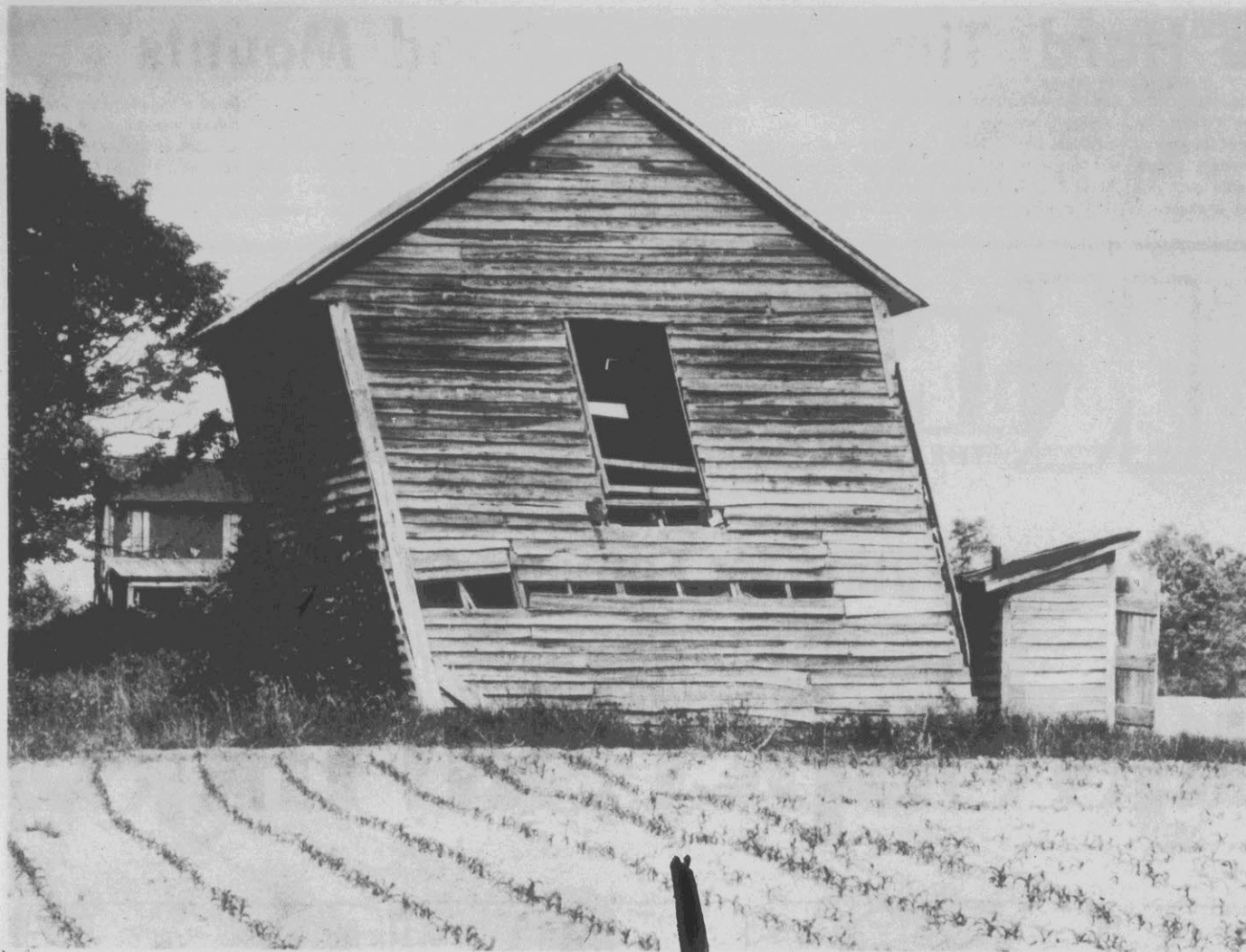
LEANING—This old barn, blown by the wind for years, has finally given away and begun leaning. Its boards are bent with time and a few are missing, here and
