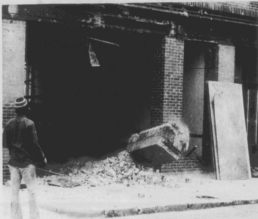
FINAL BLOWS, THEN A LEAP TO SAFETY... In the top photograph, Gary Cox delivers final blows to the base of an old brick column on the former Proctor Hotel building. In the bottom photo, Cox has leaped to a safe distance from the falling pillar, shown here just before coming to rest on the sidewalk. (Reflector Photo by Jerry Raynor)
