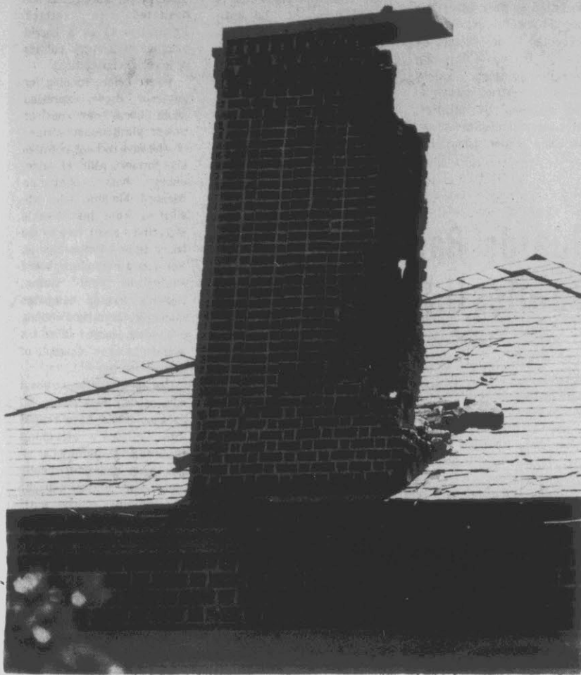
CHIMNEY DAMAGED . . . Workmen began today tearing down a chimney of Sheppard Memorial Library which was severely damaged by lightning about 7:30 p.m. Friday. Structural damage to the north end of the building called for
