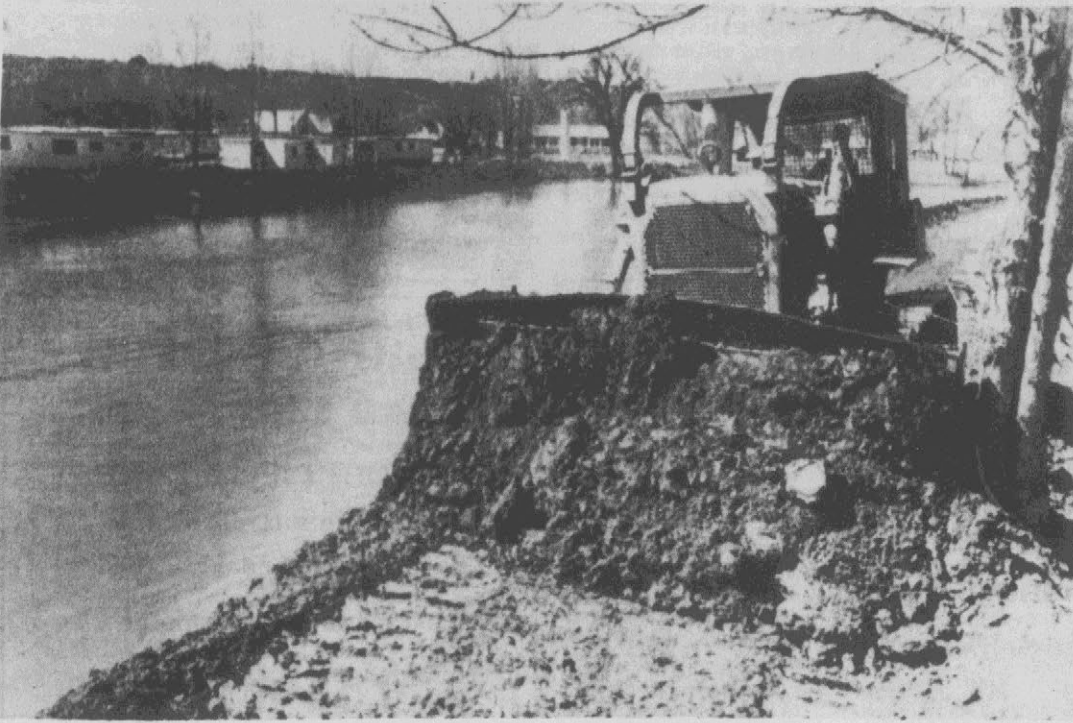
DIKING OPERATIONS — Heavy equipment moves earth along a dike holding back the swollen Sours River at Minot, North Dakota. Dike work is expected to be pressed for 24 hours a day for the next
